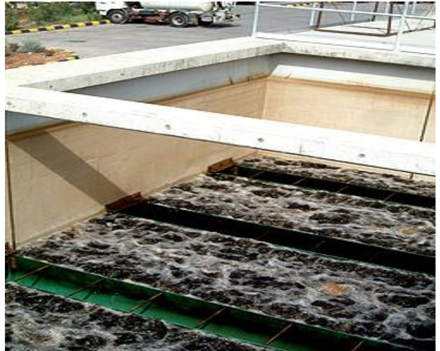
Rapid Sand Filter Back-wash and Air-wash type
