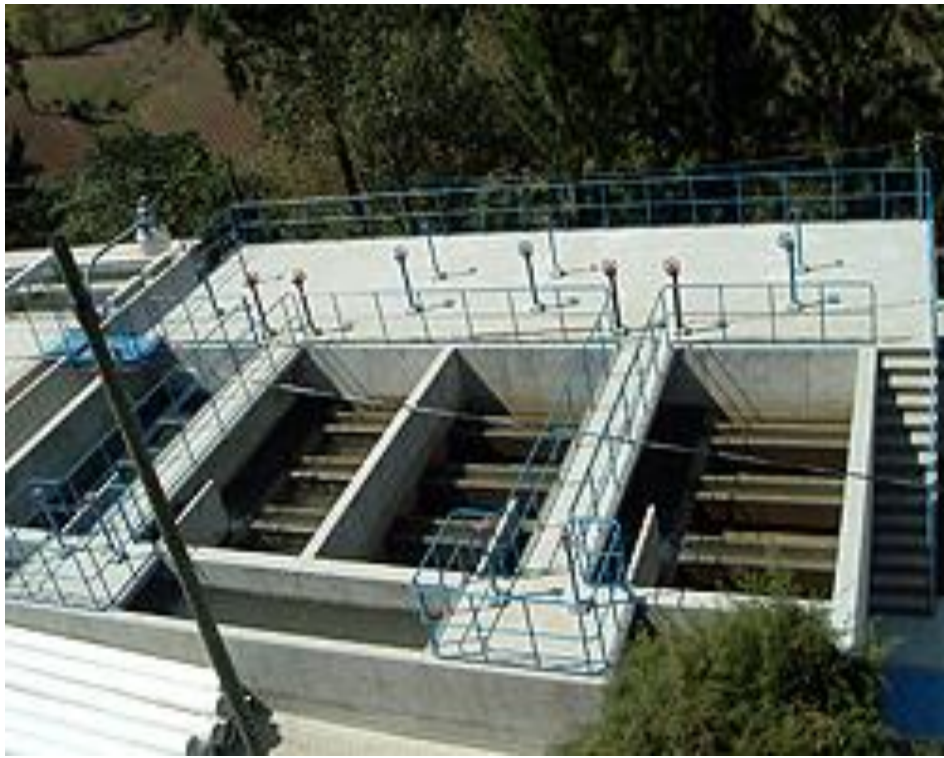
Rapid Sand Filter
