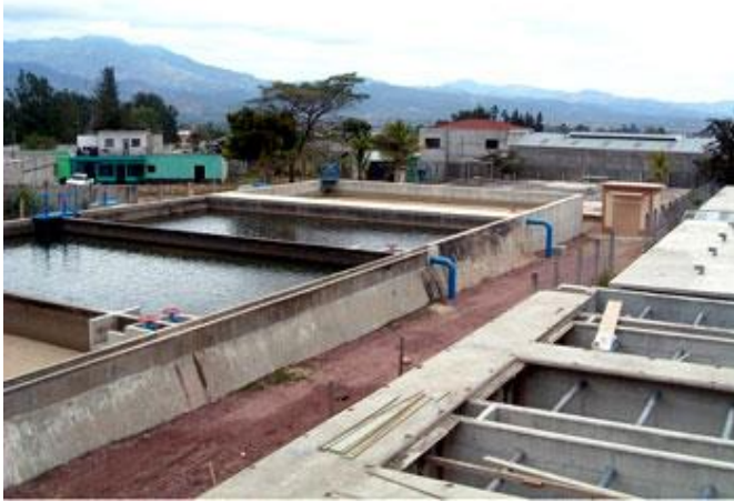
slow sand filter with water layer
